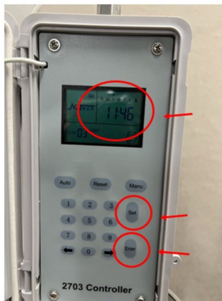
Figure 10: Manually programming the Nutech 2703 controller with the date and time.
