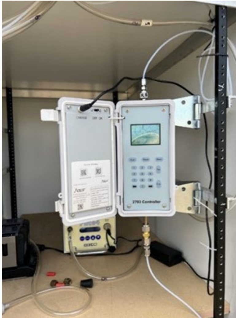
Figure 1: Nutech 2703 controller inside of a Shelter One enclosure
