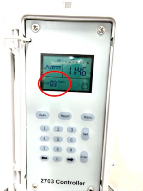
Figure 11: Manually setting the flow rate on the Nutech 2703 controller.
