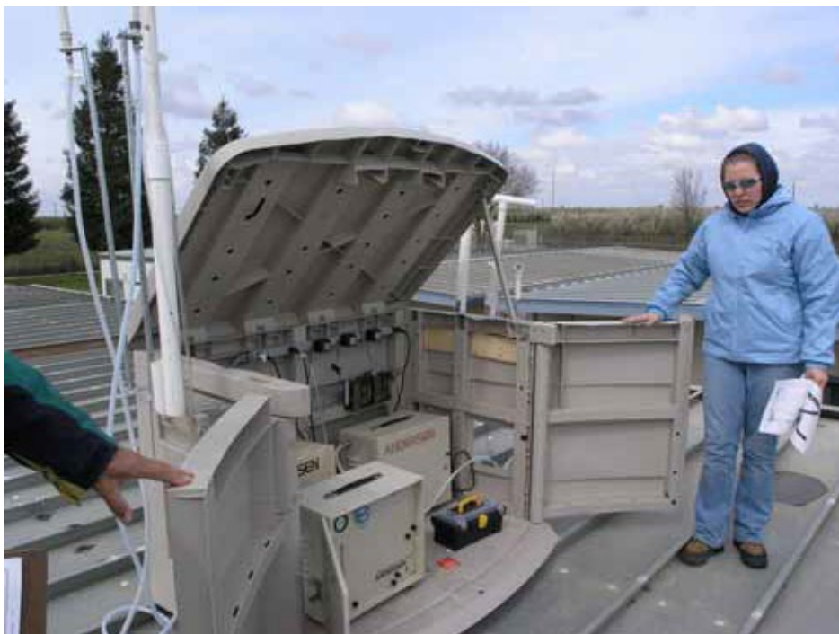
Figure 3. Air sampling equipment on a Chavez Elementary School rooftop.
