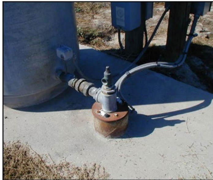
Figure 1: The well casing is the six-inch steel pipe that is slightly rusted.
