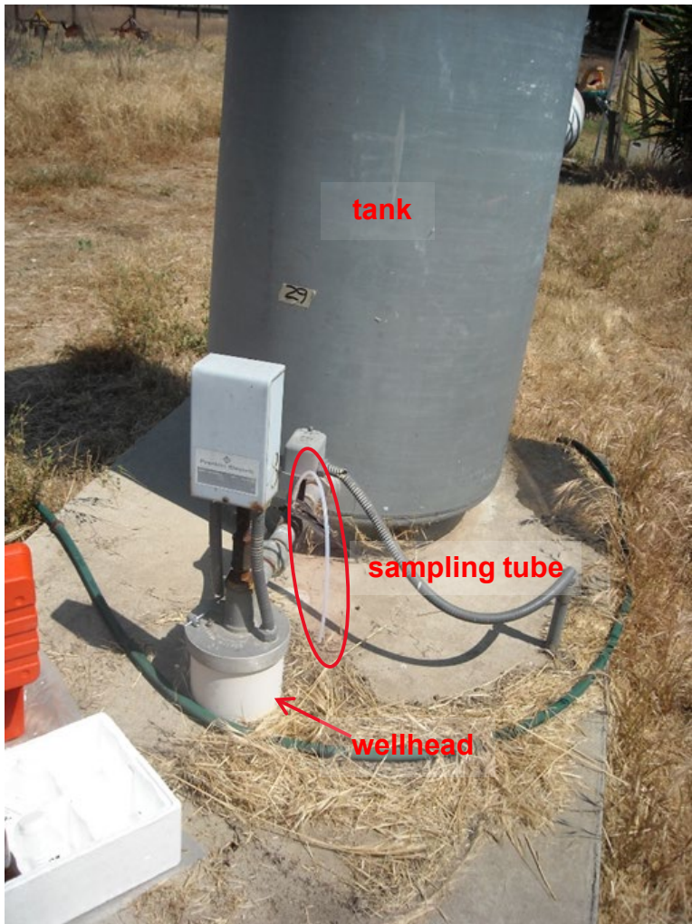
Figure 1. Well 29 sample location: A sampling tube is attached to the Schrader valve (red oval), which is between the wellhead (red arrow) and the tank
