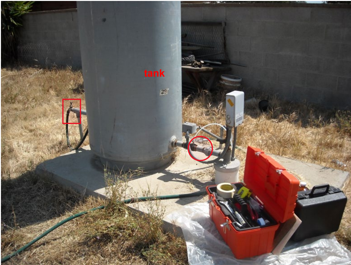
Figure 2. Overview photo of Well 29 that includes the sample location (red circle) before the tank and the faucet (red rectangle) after the tank
