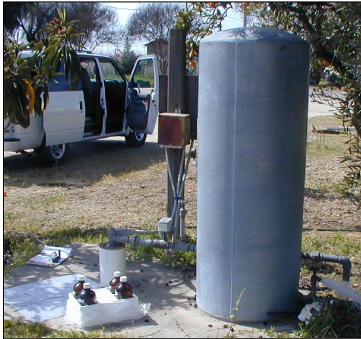
Figure 13. Example of a pressure tank. The faucet on the right is being used to keep the pump running. The faucet on the left is the best sample port.
