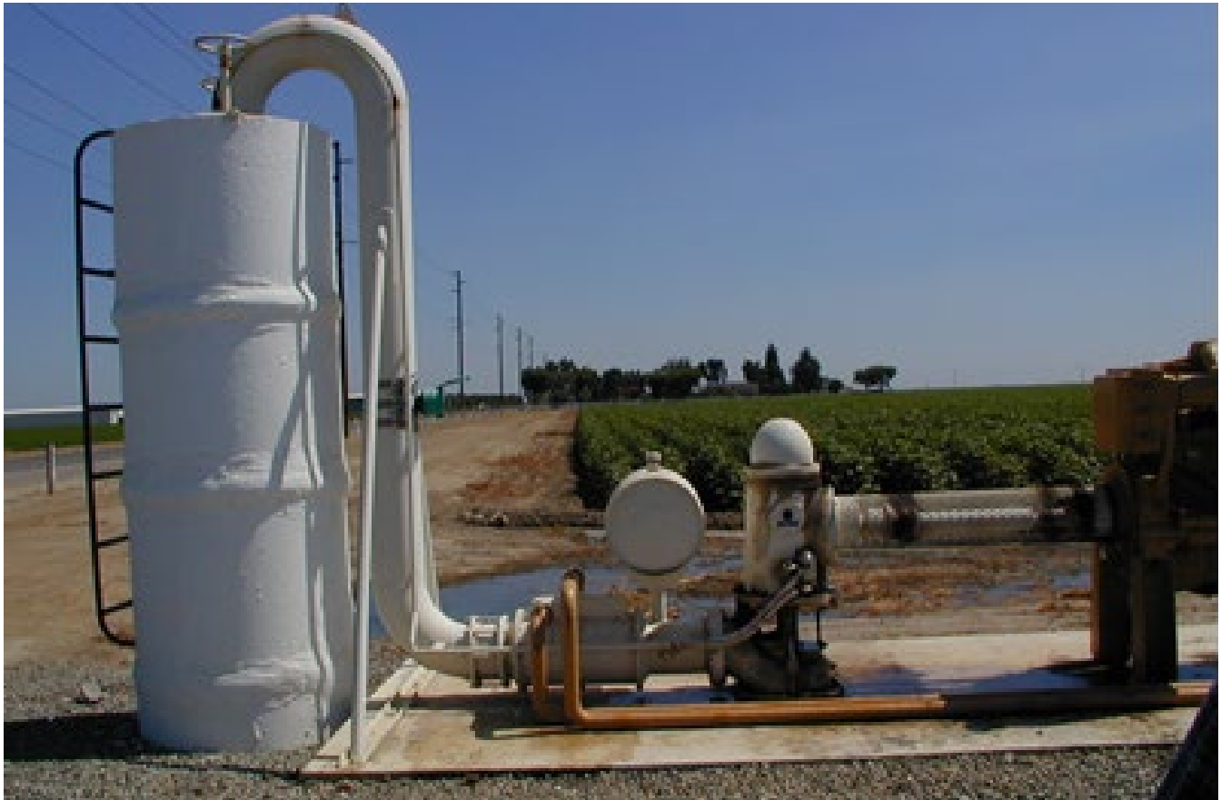
Figure 1. An example of a well with aboveground equipment and concrete pad in very good condition.
