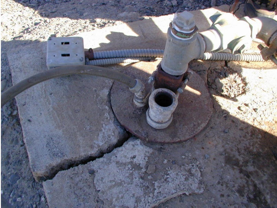
Figure 2. An example of a well in very poor condition. Note the severely cracked pad and gap at the casing. This well should not be sampled due to the potential for point-source contamination from surface water runoff.
