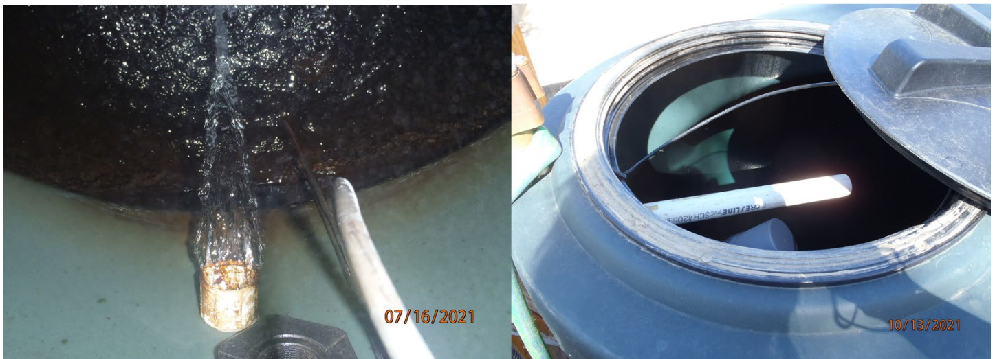
Figure 20. Left: inlet pipe inside an unpressurized tank. The black cable to the right of the inlet pipe is connected to the float valve. Right: Inlet pipe to unpressurized tank. Just in front of the pictured inlet pipe is a float valve (gray cylinder).
