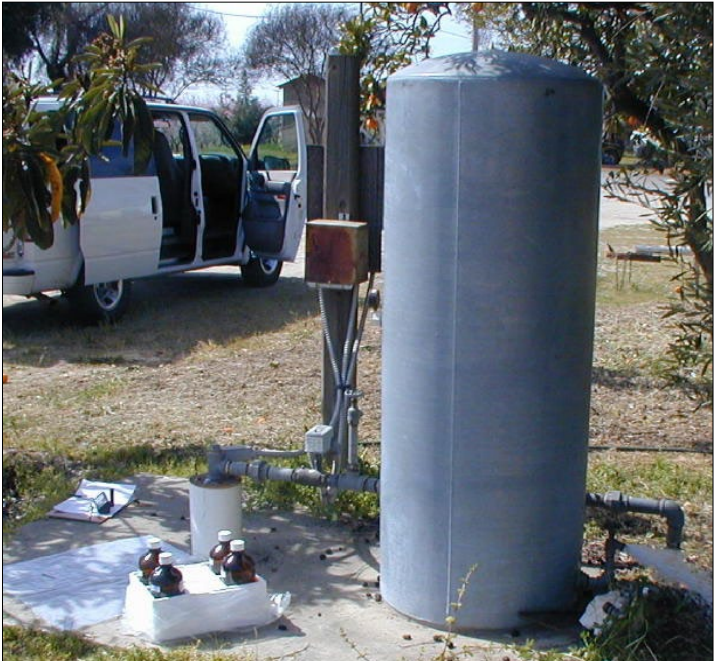
Figure 13. Example of a pressure tank. The faucet on the right is being used to keep the pump running. The faucet on the left is the best sample port.
