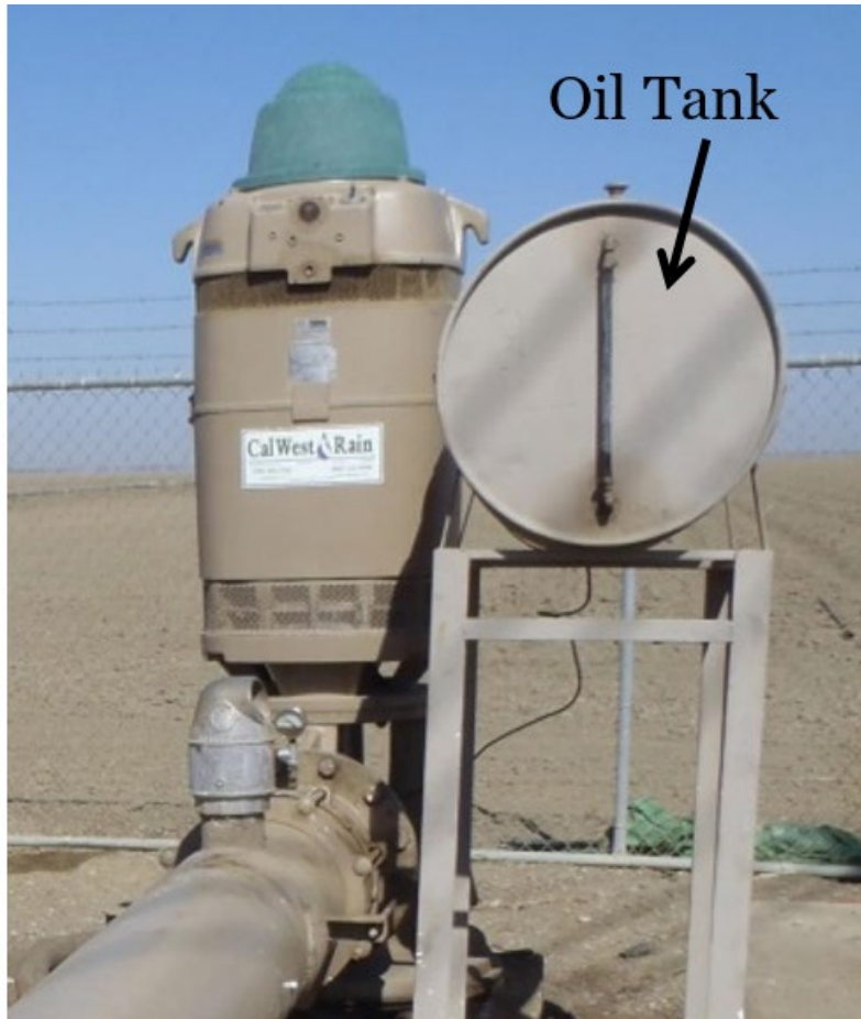
Figure 11. Oil tank for a turbine pump, not to be confused with a chemigation system.
