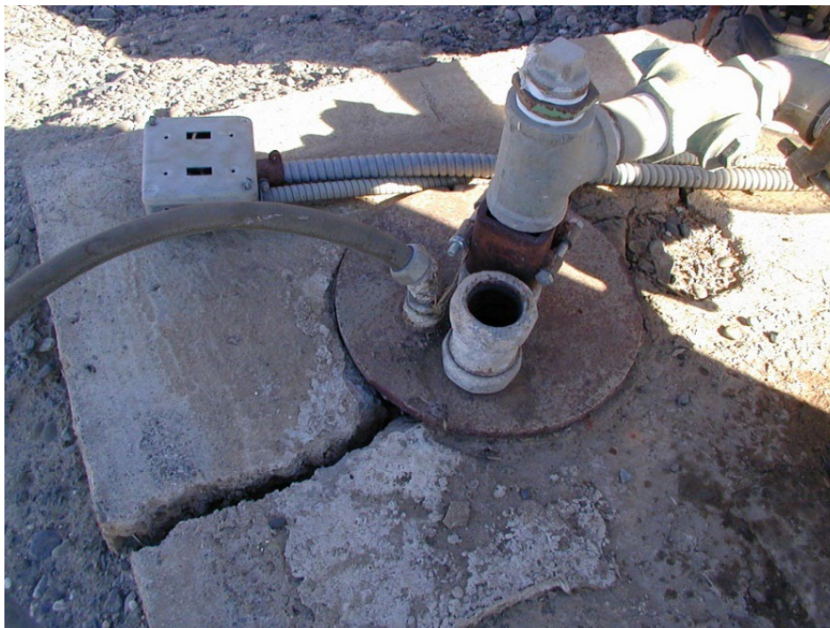
Figure 2. An example of a well in very poor condition. Note the severely cracked pad and gap at the casing. This well should not be sampled due to the potential for point-source contamination from surface water runoff.
