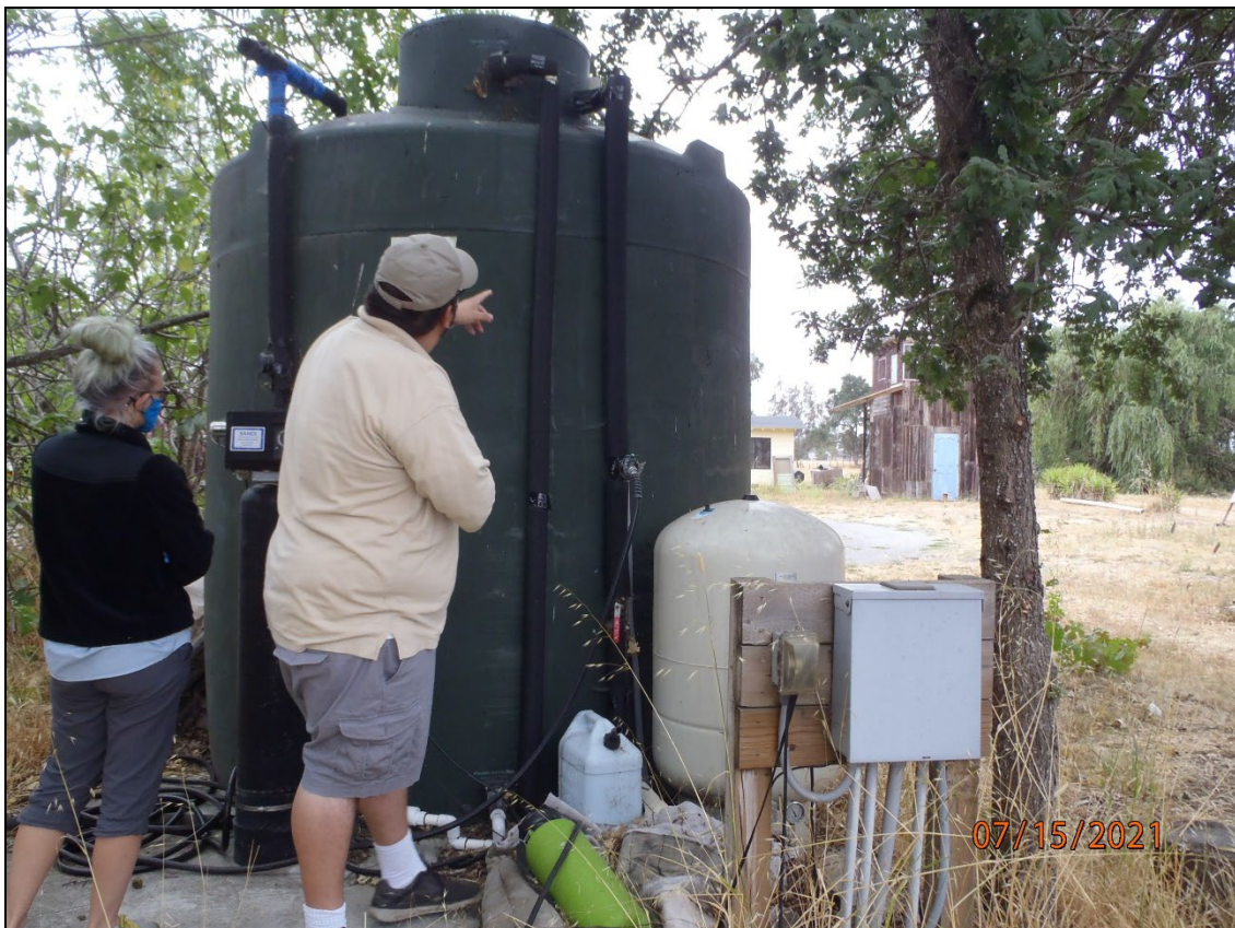
Figure 15. Example of unpressurized storage tanks. Samples were collected from the inflow into the tank from the small pipe going up the side and entering at the top by reaching inside the tank through the access port.
