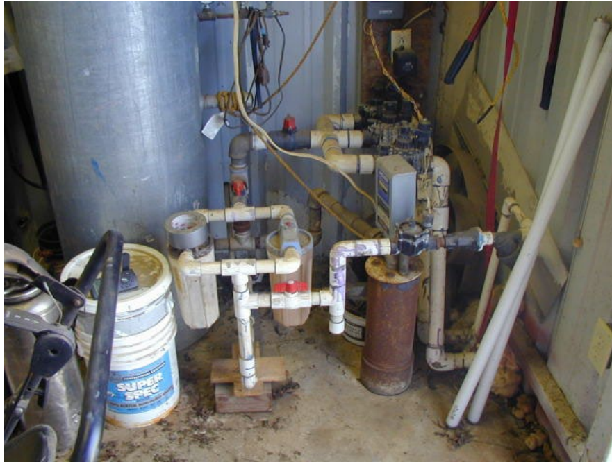
Figure 5. Locating the sampling port is not always easy. In this case, a faucet outside the shed wall to the right (not shown) could be used as the sample port as long as the proper valves were opened, negating the need to collect samples through the Schrader valve.
