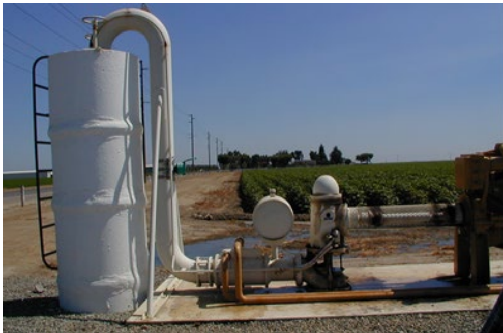
Figure 1. An example of a well with aboveground equipment and concrete pad in very good condition.
