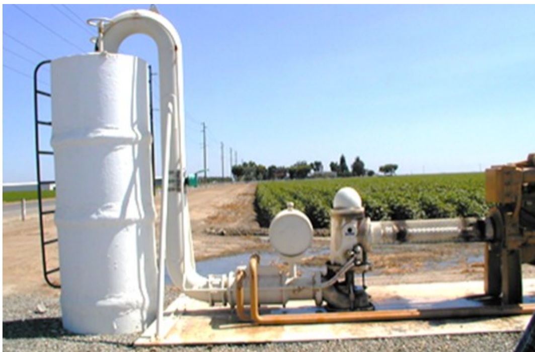
Agricultural well pumping to standpipe. Photo credit: DPR.
